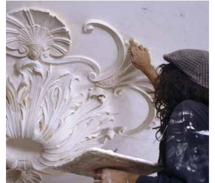
Restoration of the Staircase Hall ceiling at Uppark House and Garden following the 1989 fire
